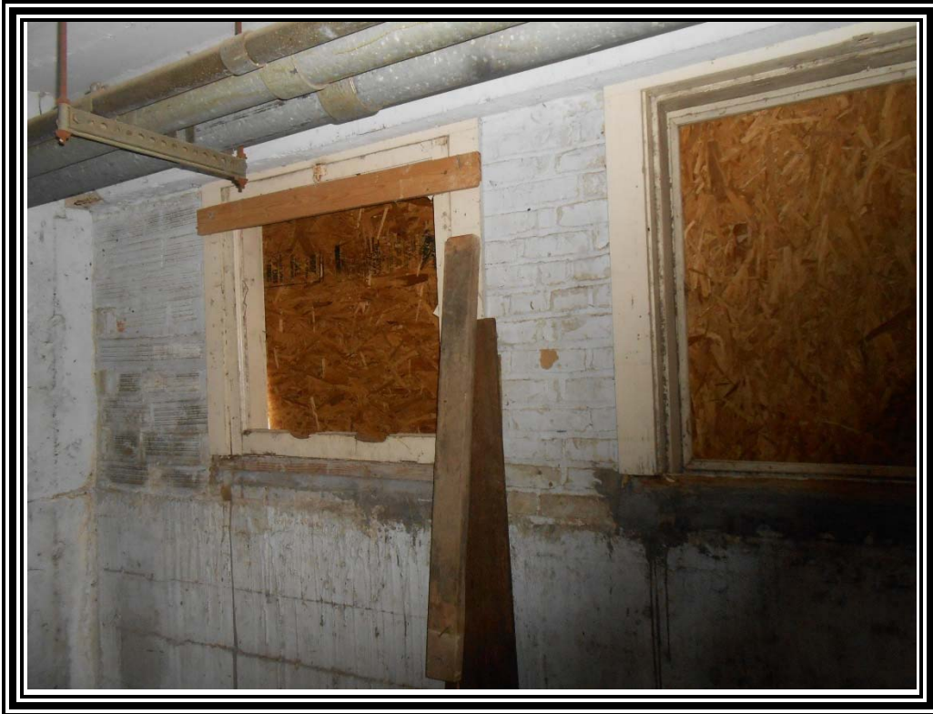
3. View of lead-containing paint on basement window frames of Drossards Hall.
