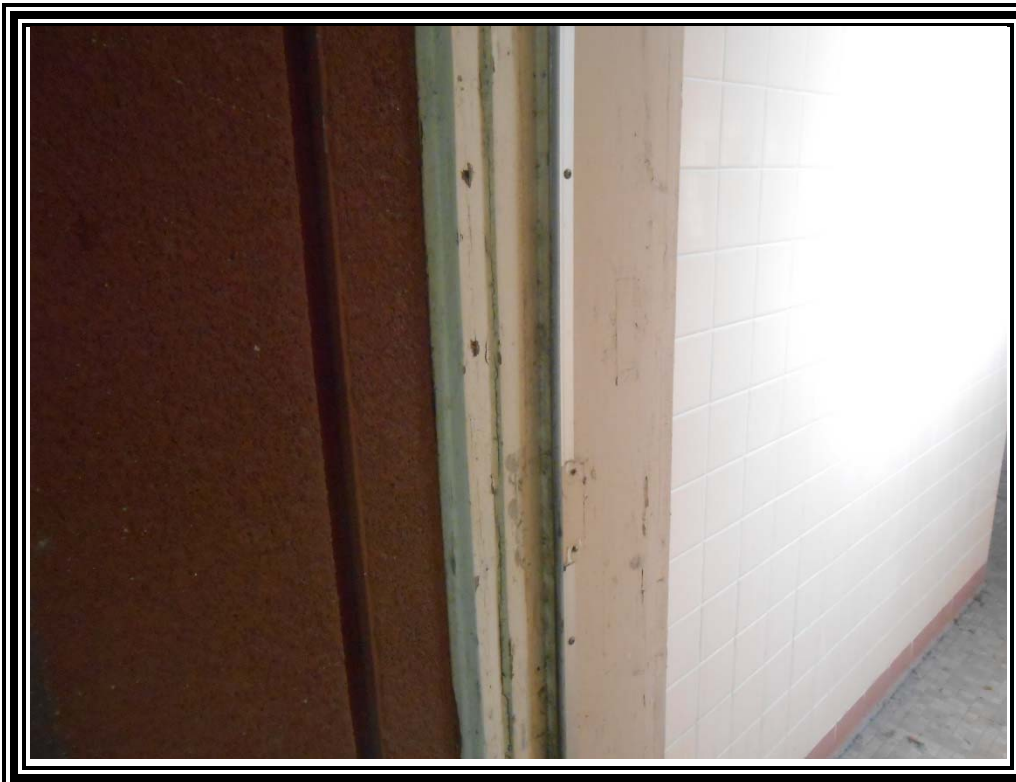
2. Door frame between restrooms and exterior of building of Drossards Hall.
