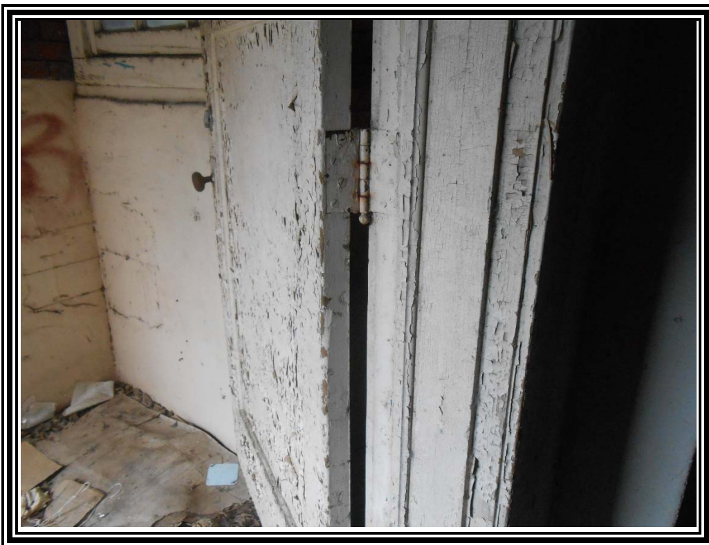
4. View of lead-containing paint on basement double door frame leading to the exterior of Drossards Hall.
